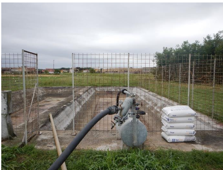
Figure 2. Tanks and sandy filters used for irrigation.
